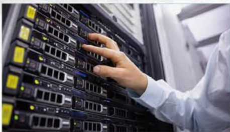
通讯设备 Automation equipment
